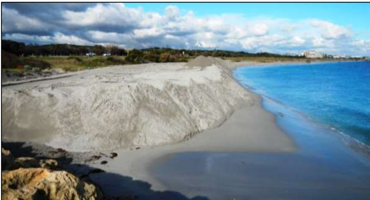
Figure 4-2 Beach renourishment occurring to protect assets at C Y O'Connor Beach, North Coogee
